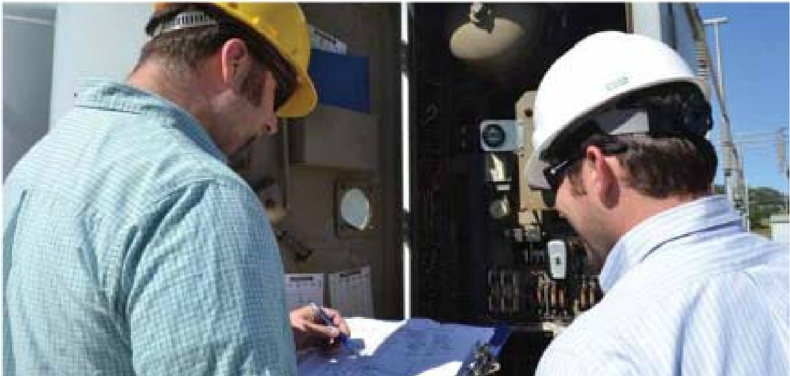
CIPCO employees Dan Dye and Craig Timson checking substation equipment ratings at Bertram substation.
